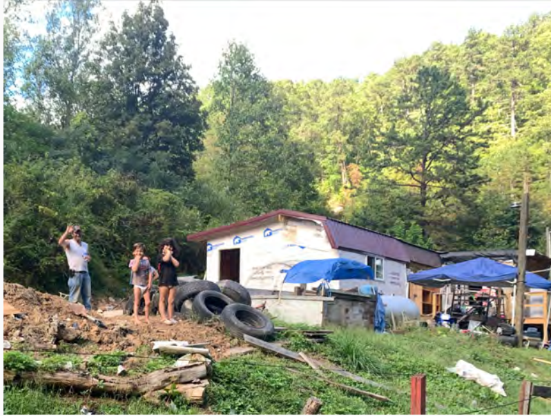
The old Martin County Courthouse also continued to receive help in their renovations through ARO's partners/teams this month! Drop ceilings were removed, furniture moved to its new locations in the courthouse, and old furniture removed from the building. We love being able to pour help back into our community!
